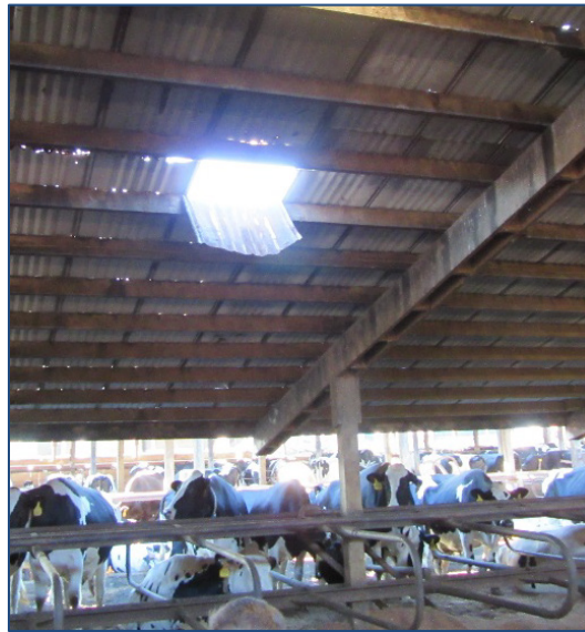
Incident scene showing the metal roof of a dairy barn through which a laborer fell 12 feet when a portion of the roof gave way. He was not using fall protection.
