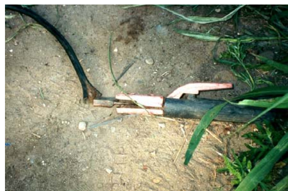
Figure 5. Un-insulated splice on bare ground
