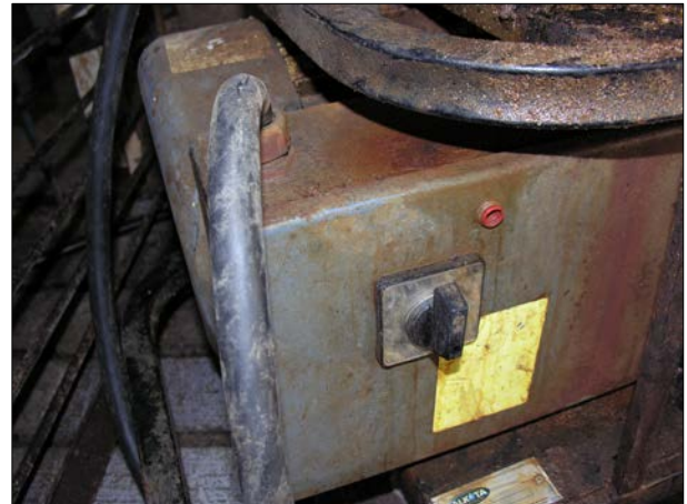
E. Cover of electrical panel box replaced in inverted orientation (above)
