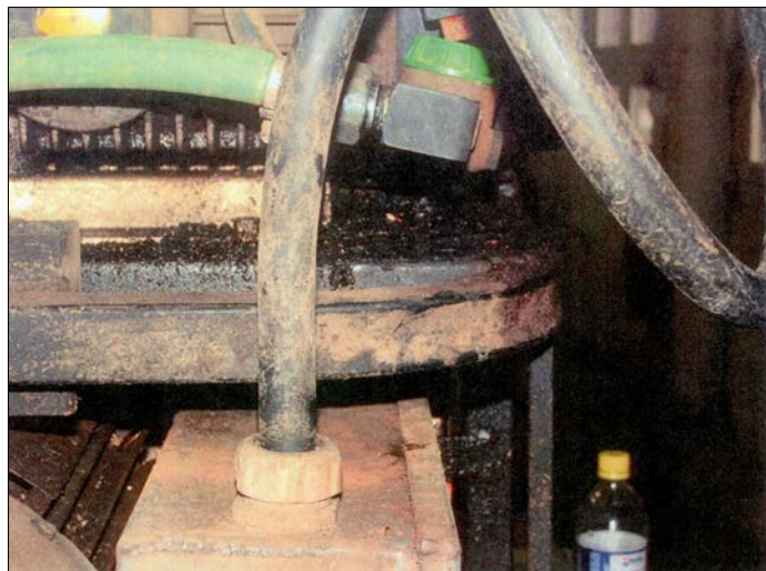
D. Water inlet located above electrical panel box (2 photos above)
