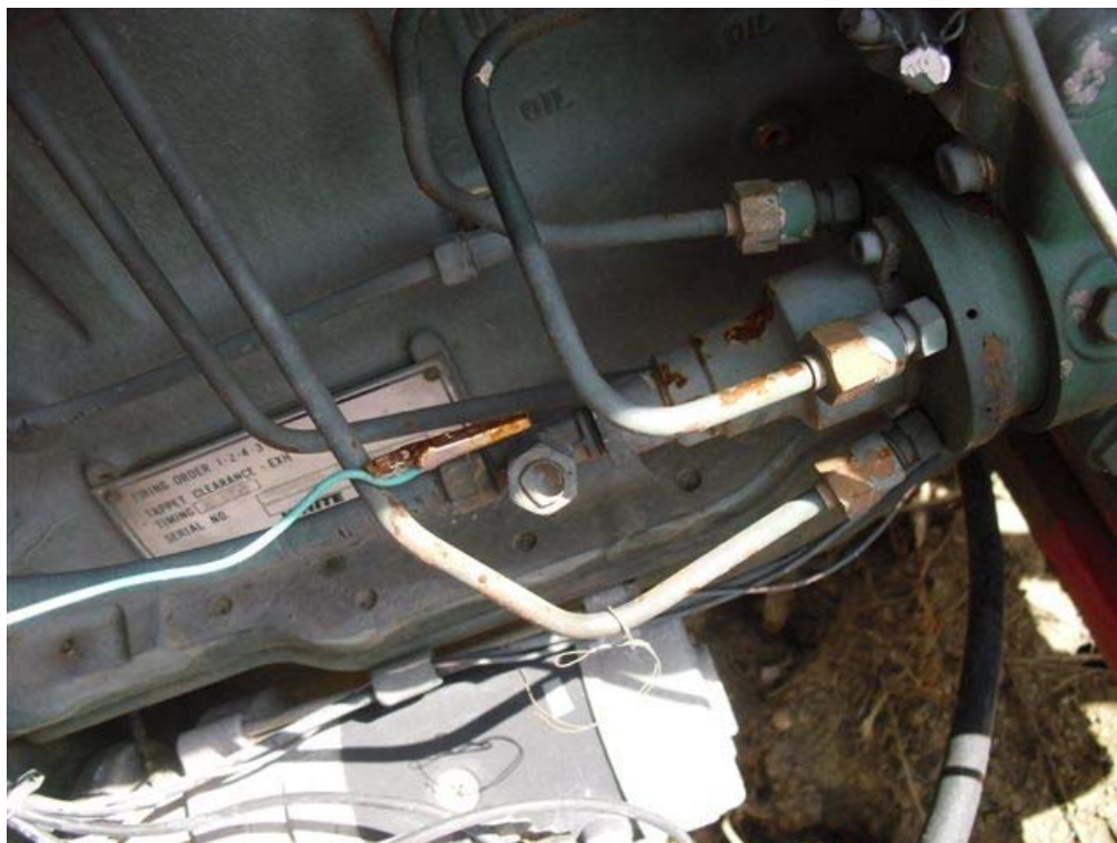
Exhibit 9. The wire clip used to shut off power to the wood chipper.
